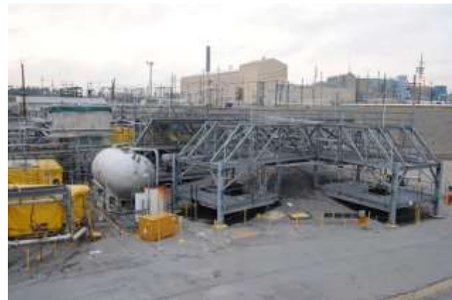
Tank 20 at the Savannah River Site
