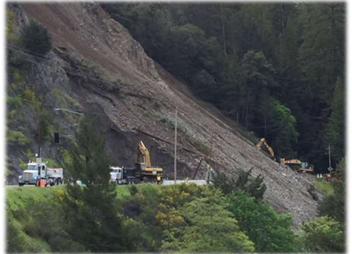
2017 Highway 101 Landslide Credit: CalTrans
